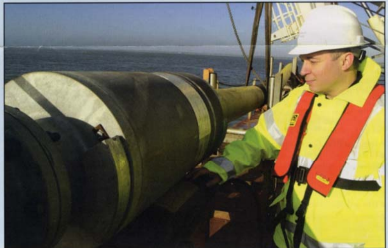
Main man: Island Manager Steve Burridge examines the new connecting joint fitted to the Cross Solent main which is being repaired to protect water supplies to the Island from the mainland
